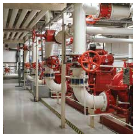
Fire Fighting Systems
