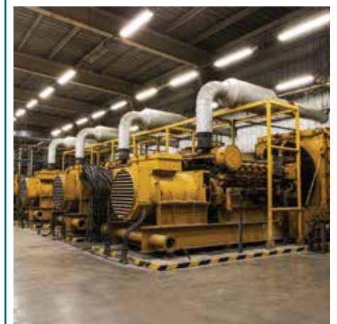
Genset & Exhaust Systems
